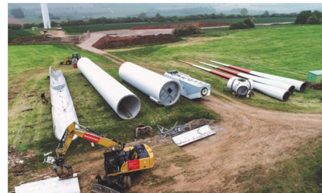
Lower image: decommissioning, energyfacts.eu
